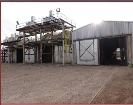
(6) STEAM FIRED ALUMINUM DOUBLE TRACK KILNS W/2022 KILN MGMT CONTROLS
